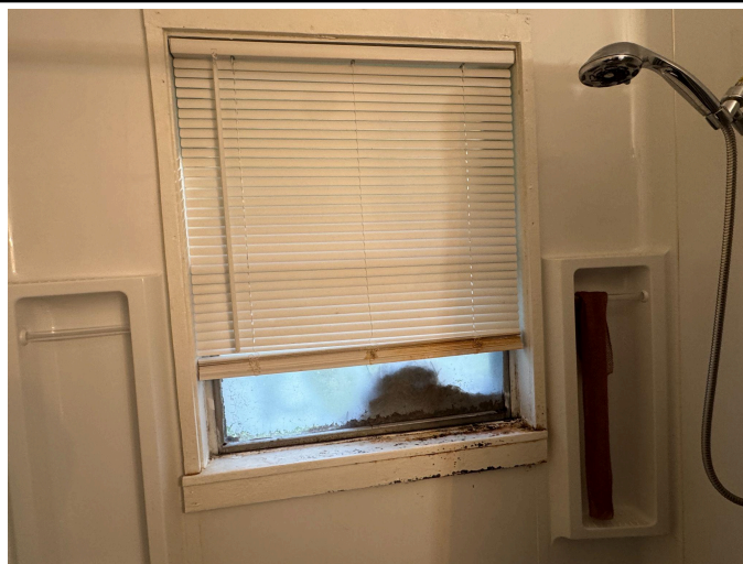
BATH 2 INTERIOR WINDOW TRIM (LBP +)
